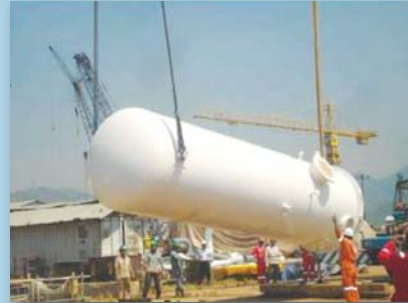
Lift and Stack Instrument Air Receiver (11-VA-0722) SCP Deck
