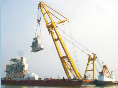
Lift and Stack Turbo Compressor 11-K 3121B
