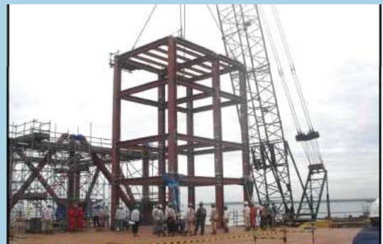
SCP pipe rack
